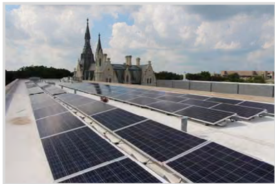
▲ Solar panel array on Kresge Centennial Hall.
