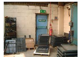
Blocked fire exit
