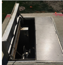
Utility Vault, Evanston
