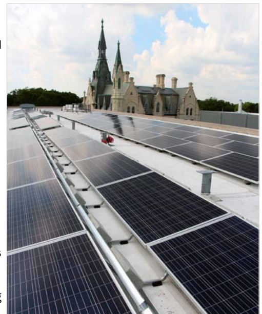
▲ Kresge is outfitted with a 254-solar panel array on the roof which is capable of generating 81 kw of electricity—enough to power 5 percent of the building's electric fixtures.
